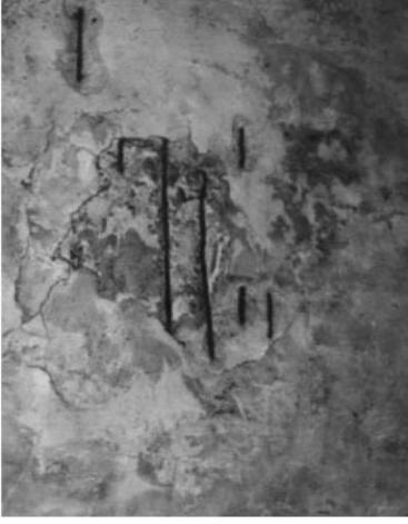
Figure 32b. Sealed ventilation openings in Crematorium I ceiling. It is not known why some rebar crosses opening.
