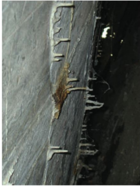
Figures 20a, b, and c. Three of the indentations in the gas chamber ceiling; in 20b (center), rusted rebar just touches inner edge; in 20c (bottom), wood block survives.
