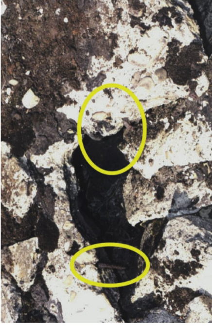
Figure 14. Inwardly bent rebar at north and east edges of second Zykion hole, partially destroyed in explosion.
