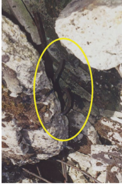
Figure 13. Straight edge and inward-bent rebar on southern side of second Zykion hole. Such bending could not result from the explosion, which lifted the roof upwards.
