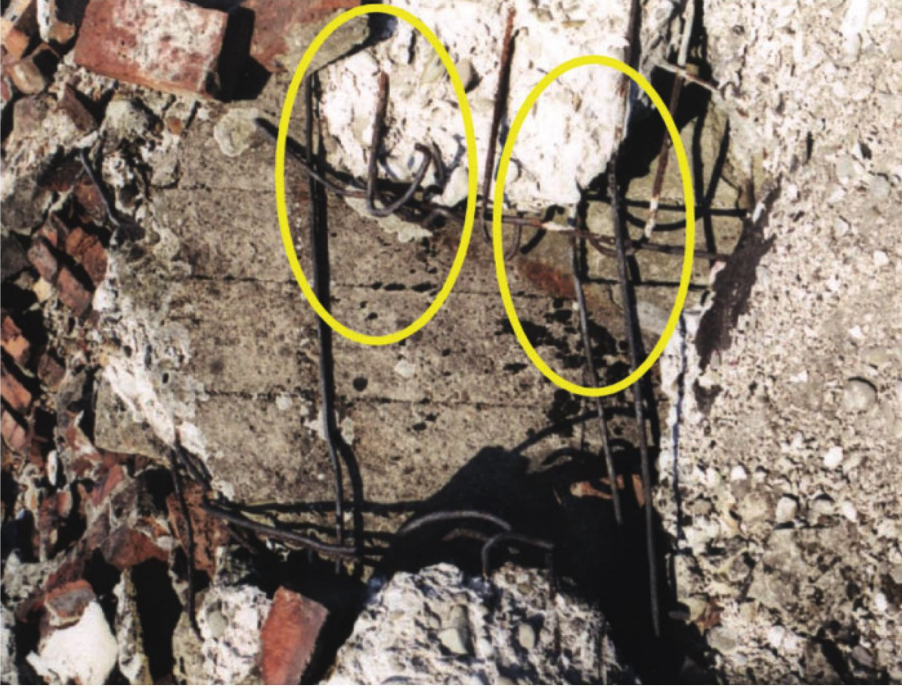
Figure 16. Remains of fourth (seen from south) Zyklon hole. Rebar skirts two sides, ends at other two sides bent inward and looped back. Note rotated roof slab showing formwork on inner side.
