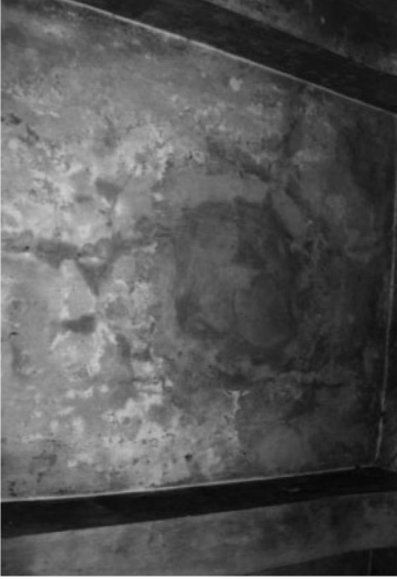
Figure 31. Sealed Zyklon hole Z1, which was not reopened during post-war restoration. Photograph taken inside chamber. It is not possible today to see the sealing signs on the roof, which was covered with heavy tarpaper.
